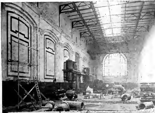
FIG. 3.—INTERIOR OF NEW PORTION, BOSTON EDISON PLANT.
